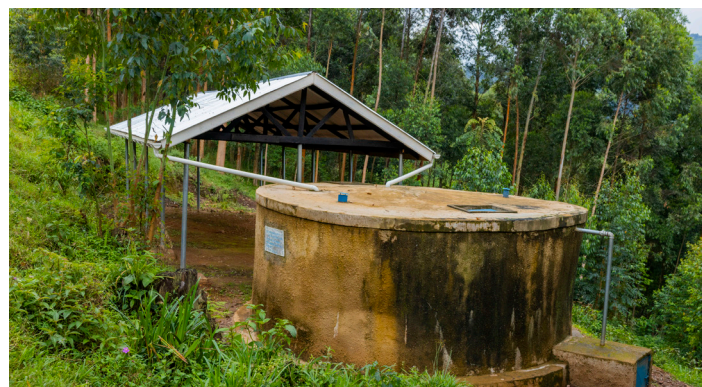
A 30m 3 rainwater harvesting tank with a roof catchment in Nyarusuzu.
